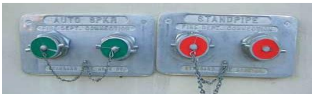
Figure 4-11. Fire Department connections serving a sprinkler system protecting an entire building or structure shall be provided with caps painted green. (left)
