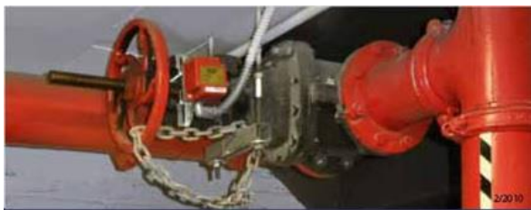
Figure 4-9. This OS&Y control valve is locked in open position.
