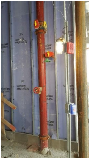
Figure 4-2. Standpipe at Construction Site
