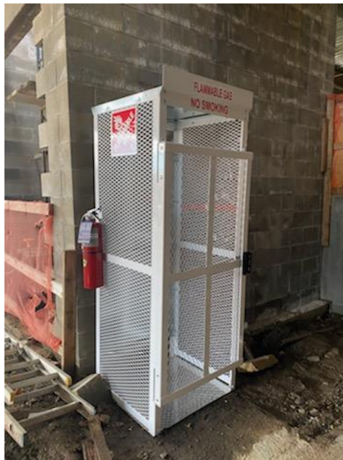
Figure 8-3. Acceptable storage enclosure.
