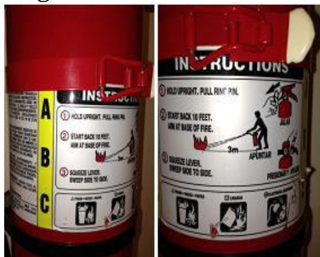
Figure 5-7. ABC Fire Extinguisher Label
