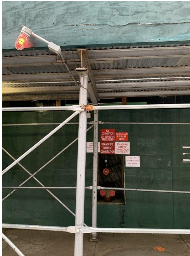
Figure 4-4. Proper sign and red light provided at the FDNY connection
