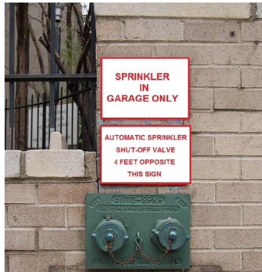
Figure 4-13. Fire Department connections serving a sprinkler system protecting only a portion of a building or structure shall have durable metal signs securely fastened to, or above, the connection indicating the portion of the building or structure protected.
