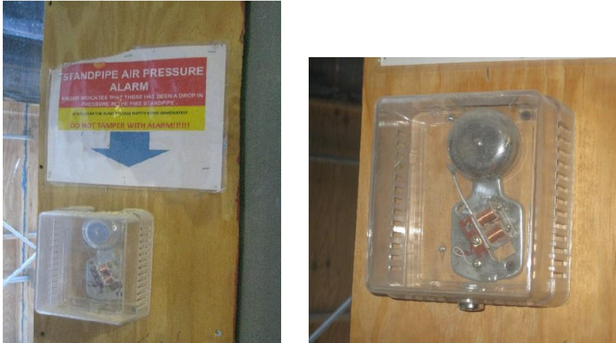
Figure 4-14. Standpipe alarm system
