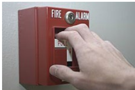
Activating a single action station
